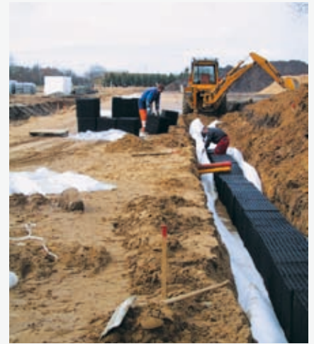
Longitudinal drywell, residential area
